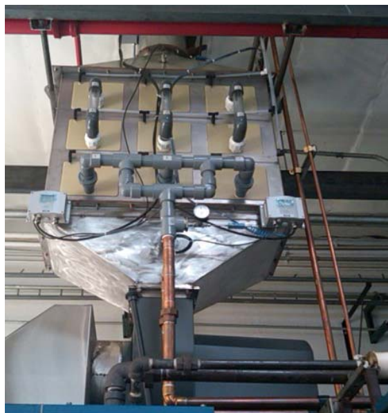
TMC installed on top of the steam tunnel at L.&N.
